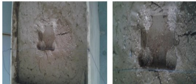
Fig 21 -After removing the plate appearance of the soil
