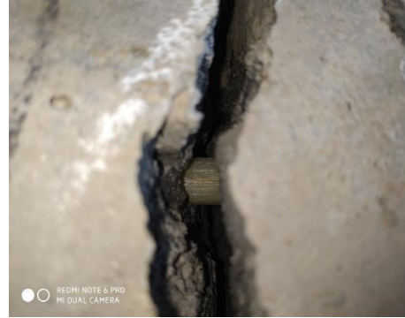
Fig. 3: Crack pattern of beam
