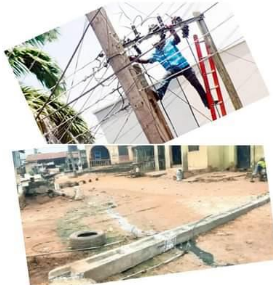
Fig 2: Unexpected Peril: A Utility Worker's Fall During Routine Maintenance in Abule, Arepo.
